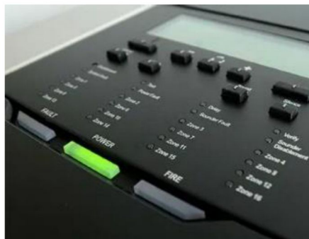
Voice Alarm/PA Systems
