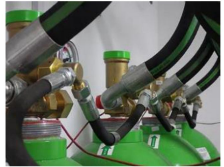
Fire Suppression Systems
