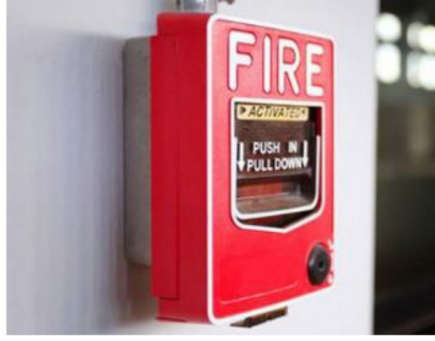
Fire Alarm Systems
